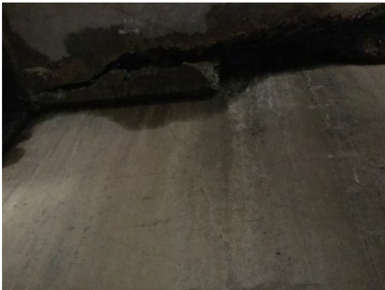
Damage to panel 1 at right bank
