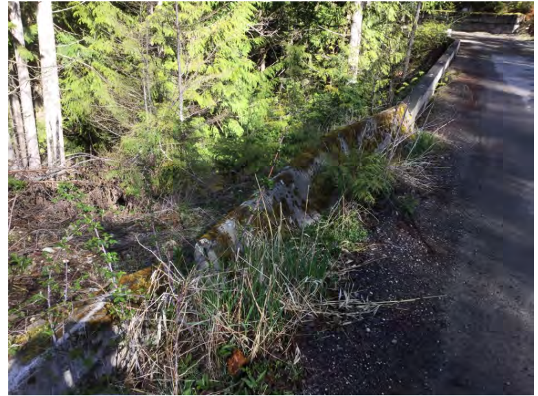
No post barriers falling off road and or unconnected
