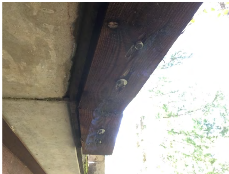
Missing washers on rail bolts
