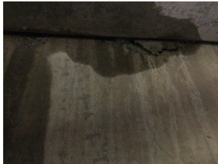
Damage to ballast wall at right bank
