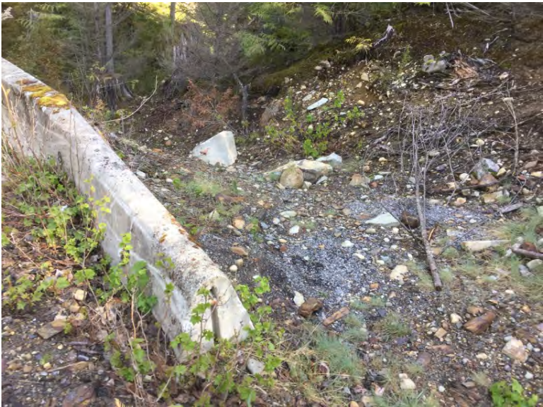
Missing bullnose at upstream left bank
