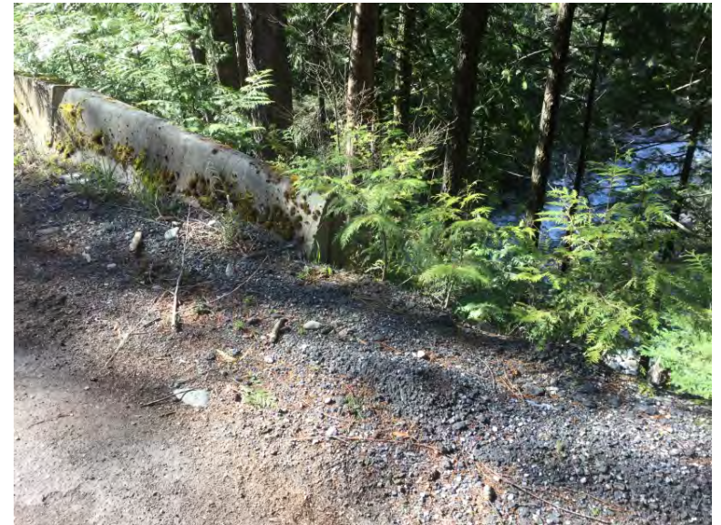
Missing bullnose at downstream right bank, it's over the bank
